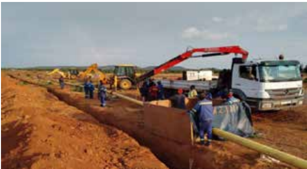
Construction of the new three (3) kilometre pipeline from the main line to Mpika Depot
